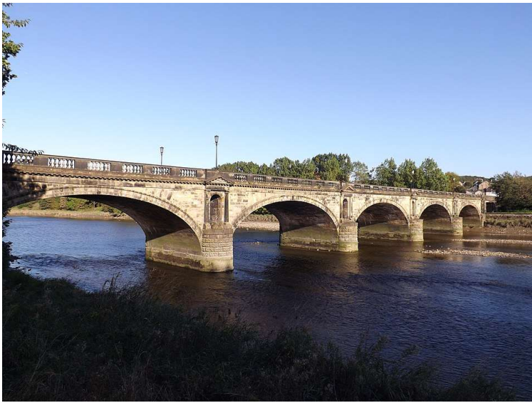
In 1839 he supervised the repair of Skerton Bridge over the River Lune
